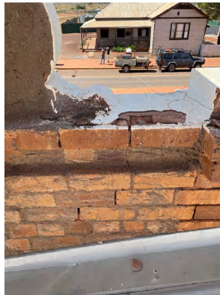
Plate 49 – Previous repairs to parapet, crack propagating through
