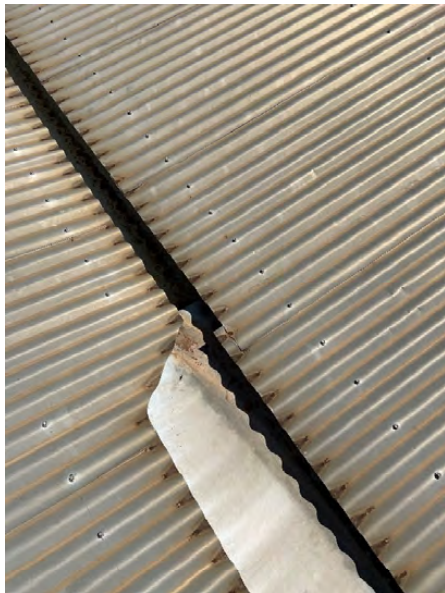
Plate 56 – Transition in box gutter to deeper but thinner section
