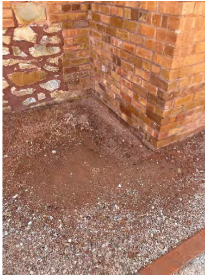
Plate 18 – Unsealed area adjacent to foundations, visible moisture to lower masonry and efflorescence indicating rising damp
