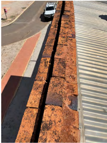
Plate 51 – Missing capping brick and slight rotation of external leaf of parapet
