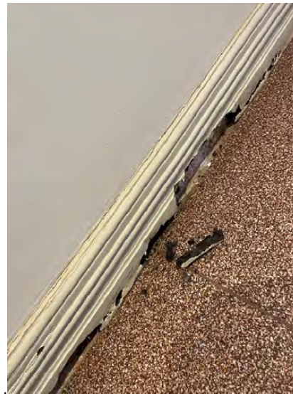
Plate 35 - Water ingress to skirting below box gutter
