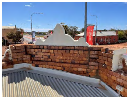
Plate 45 – Lower parapet previous repair, soft mortar
