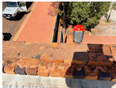
Plate 50 – Deterioration of capping mortar
