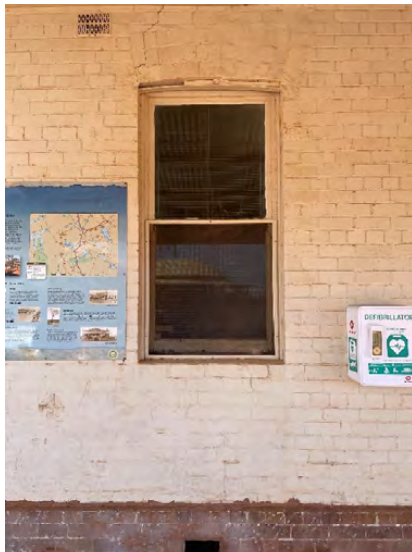
Plate 2 – Cracking to masonry arch and painted fascade
