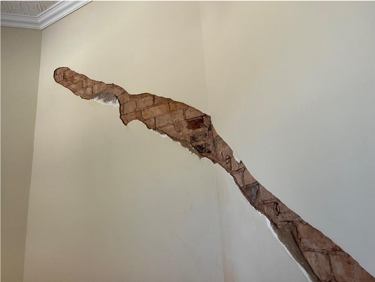
Figure 1: Diagonal Cracking in Central Corridor
