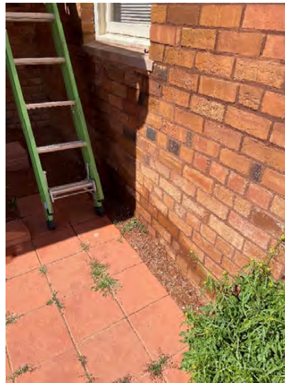
Plate 12 – Visible moisture to lower masonry and efflorescence indicating rising damp
