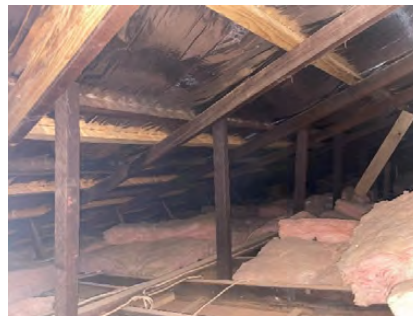
Plate 40 - Previous augmentation of roof framing
