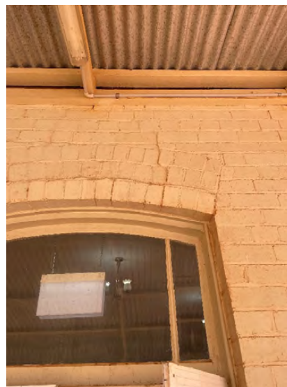
Plate 4 - Cracking to masonry arch
