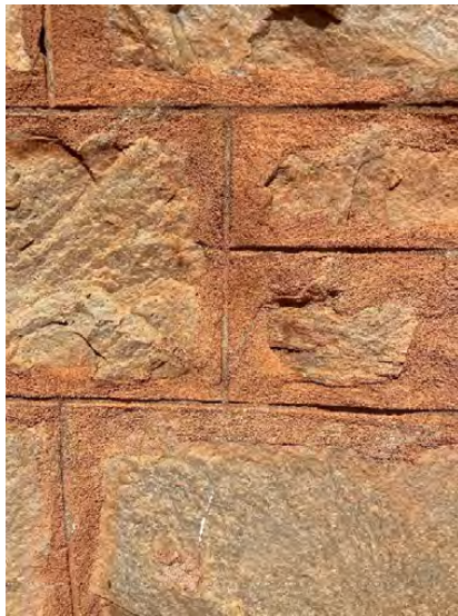
Plate 6 – Hard mortar (possibly with cement)
