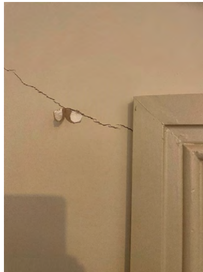
Plate 39 - re-entrant cracking to plasterboard
