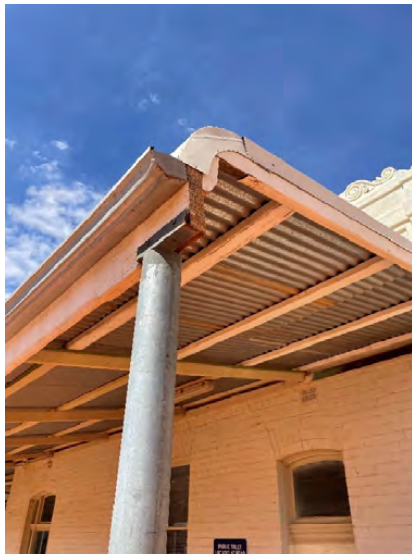
Plate 9 – Poor tiedowns/connection to veranda post
