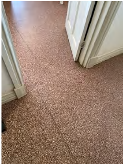
Plate 38 - Displacement between infill concrete panels
