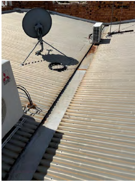
Plate 55 – Shallow box gutter and evidence of pooling
