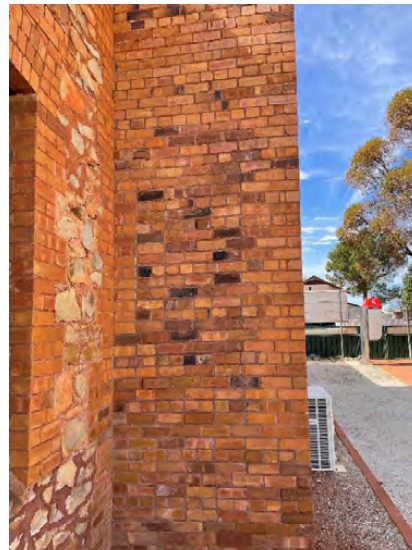
Plate 16 - Cracking to external masonry, slight rotation of return wall
