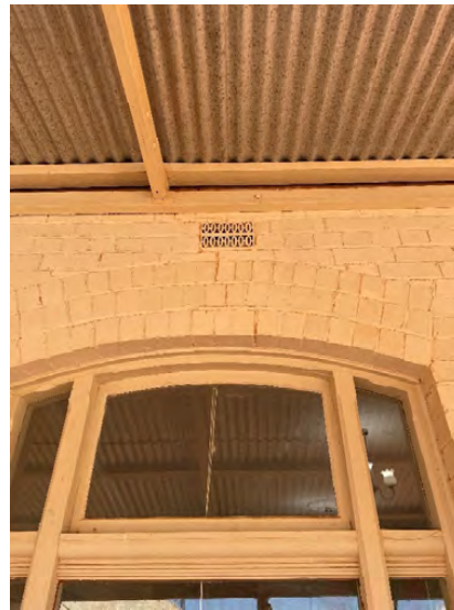
Plate 3 - Cracking to masonry arch
