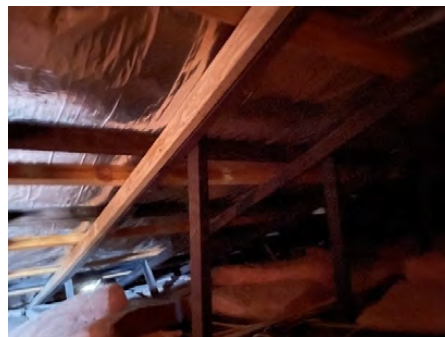
Plate 41 - Limited tiedowns noted
