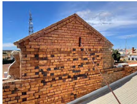
Plate 44 - Façade Parapet poorly braced, soft mortar
