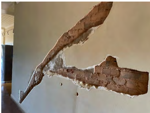
Plate 26 - Proposed repair location
