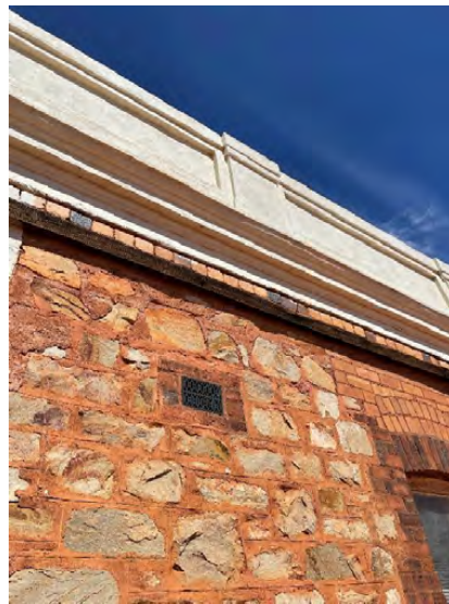
Plate 8 – Hard mortar (possibly with cement)
