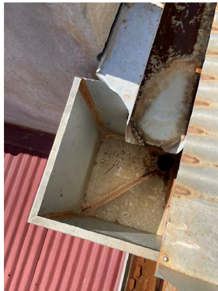
Plate 58 – Box gutter discharge, no provision for overflow, small diameter downpipe
