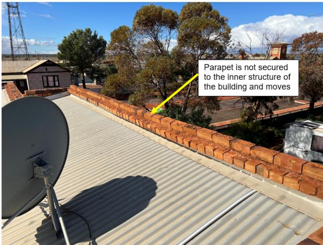
Figure 6: Southern Parapet not tied into Internal Building Structure
