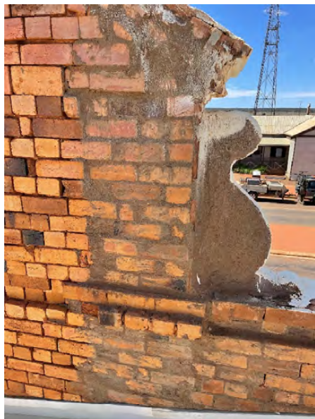
Plate 48 – Soft mortar and previous repairs to parapet
