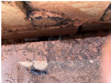
Plate 52 – Missing capping brick and slight rotation of external leaf of parapet
