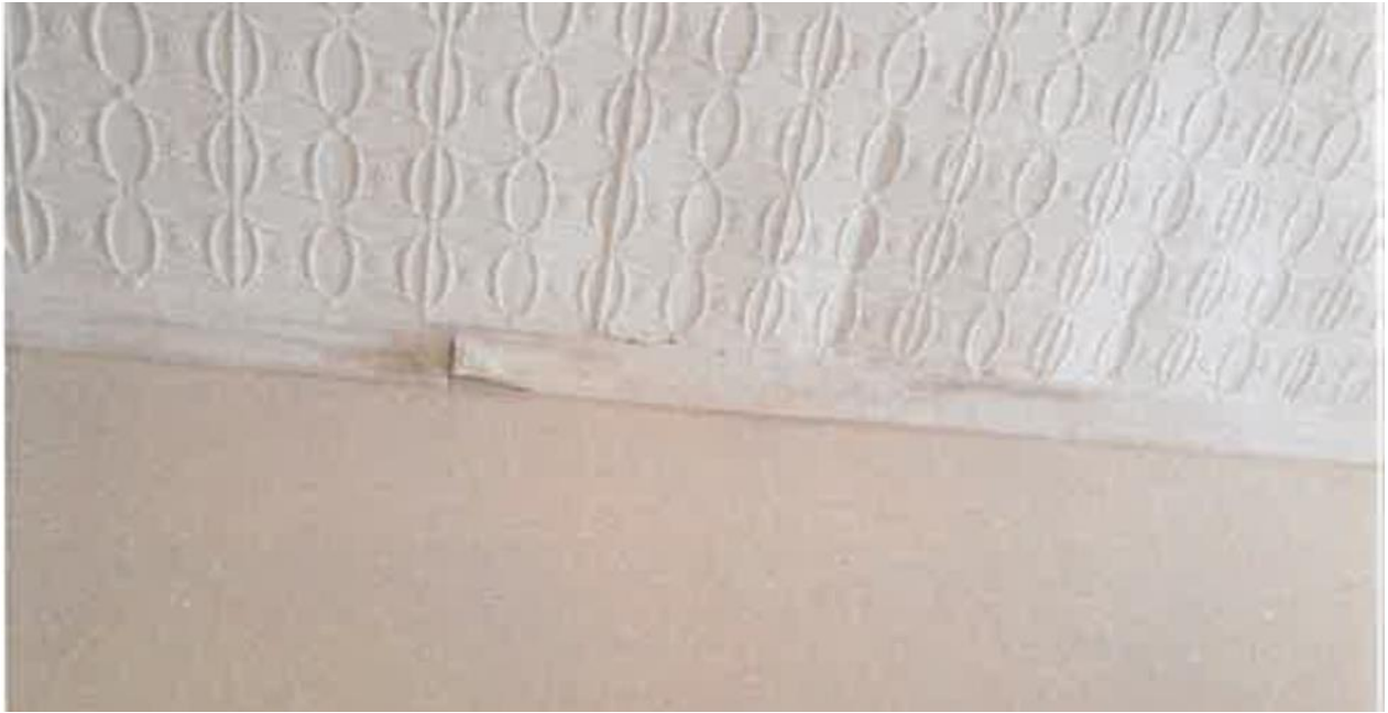
Figure 3: Roof leak from undersized box gutter
