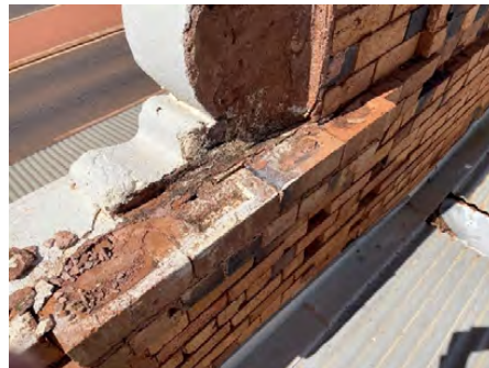
Plate 46 – Capping mortar missing
