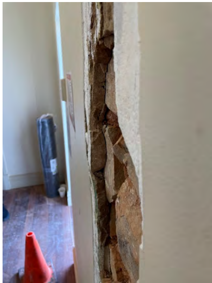
Plate 22 - Proposed repair location
