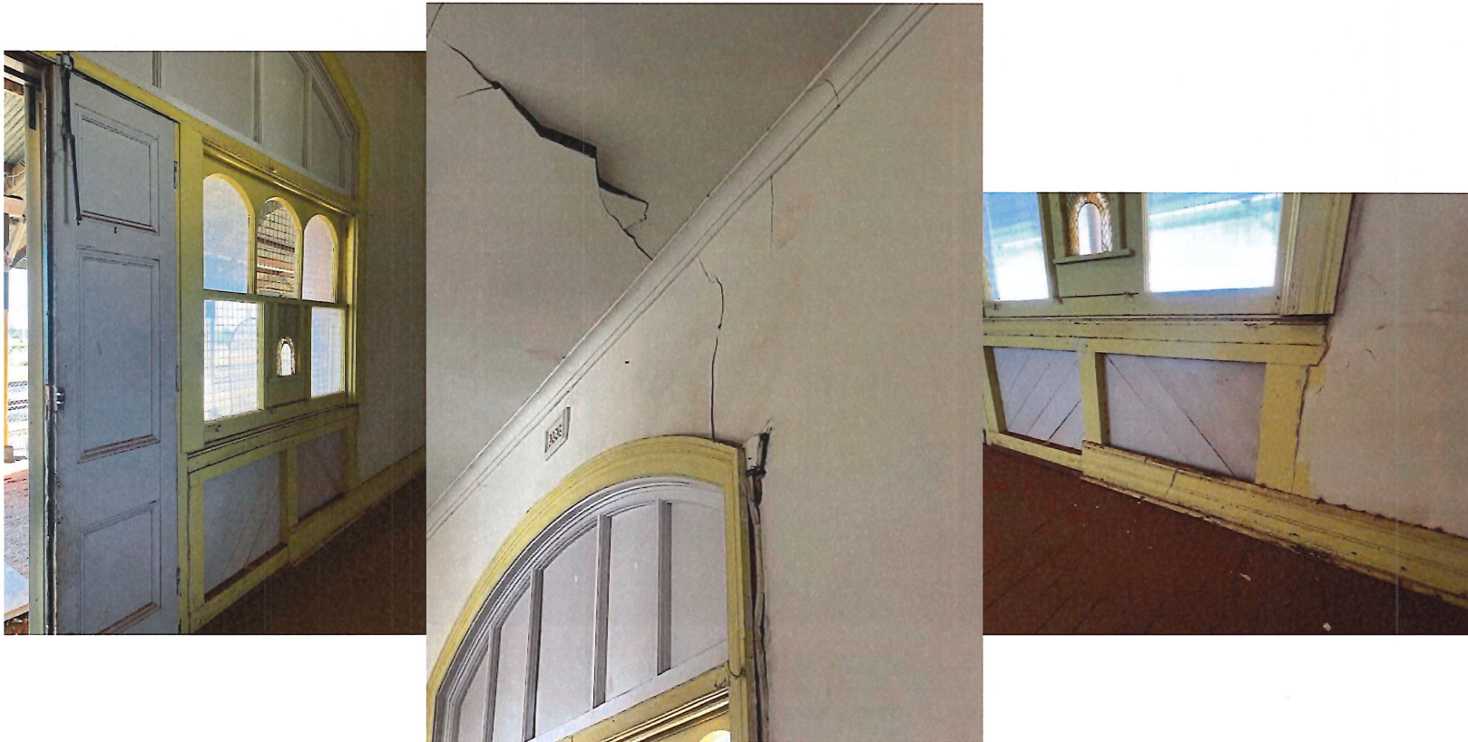
Photos 60, 61, 62 Interior: Luggage room showing arched window set, damage to wall and ceiling and at dado level.
