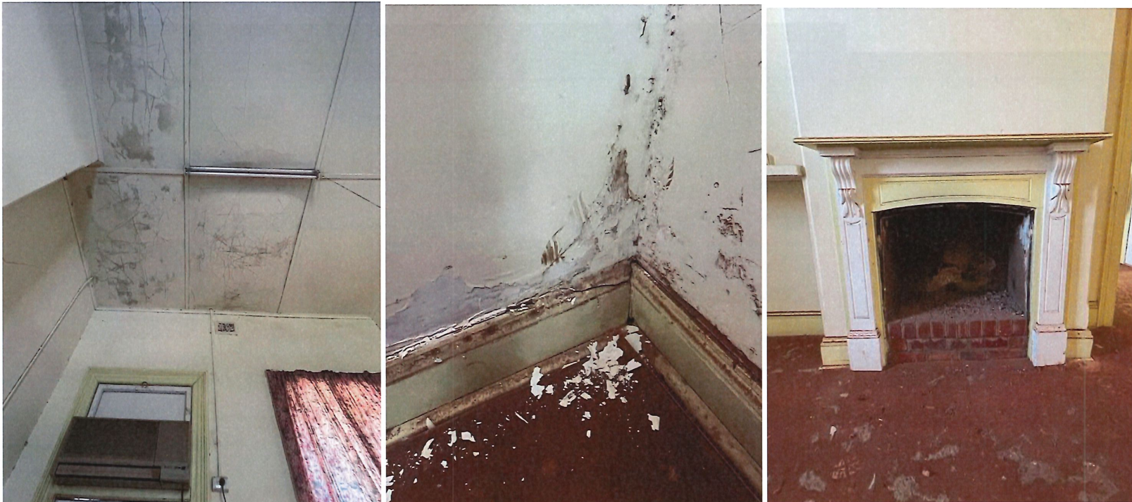
Photos 80, 81, 82, 83 Interior: Stationmaster's room showing moisture damage to the ceiling in the northwest corner, moisture damage on the lower wall in the southeast corner, and the intact fireplace on the north wall.
