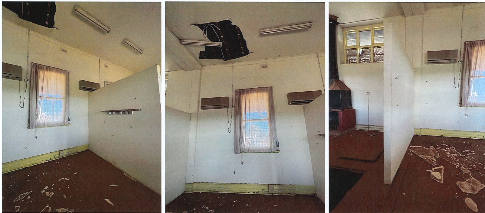
Photos 63, 64, 65 Interior: Luggage room showing timber framed partiitons and ceiling damage. The second partition is where the original wall between the luggage room and refreshment room was located.
