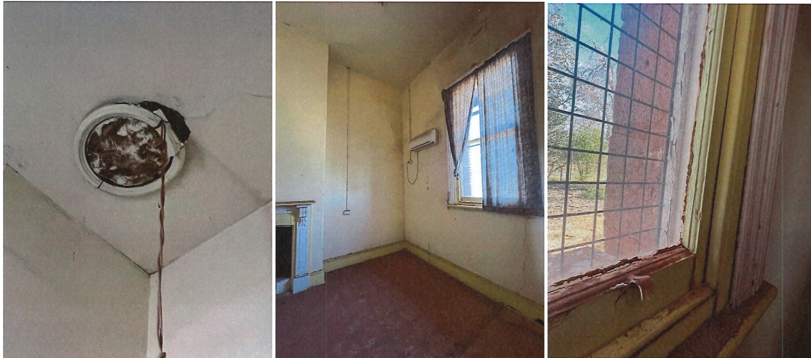
Photos 47, 48, 49 Interior: Ladies room partitioned section on the west side- damaged ceiling vent, west frontage window, and window frame detail.
