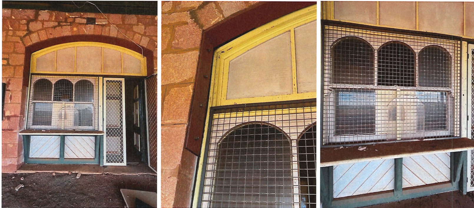
Photos 25, 26, 27 The arched window set, showing steel structural reinforcement, and pair of paneled entry doors into the luggage room off the railway platform.
