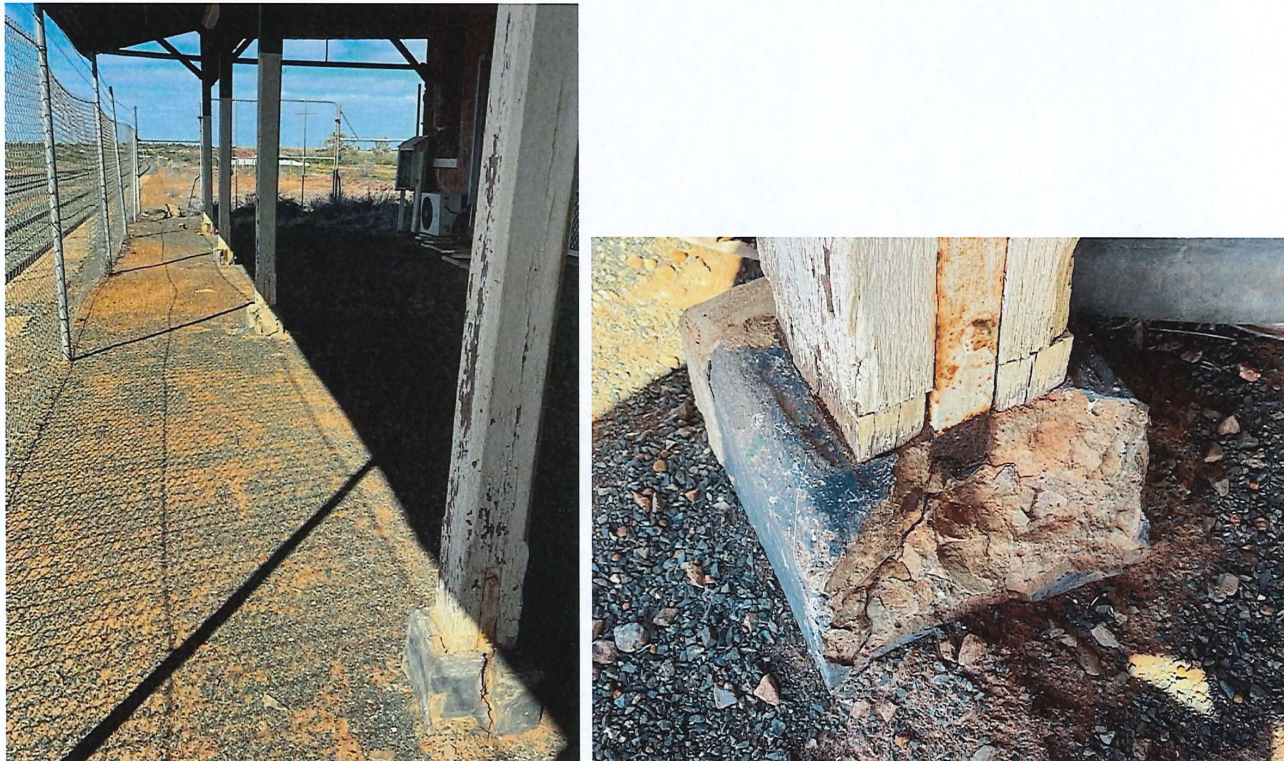
Photos 36, 37, 38 View looking south down the platform showing the damaged posts, and details of damaged deteriorated veranda posts (typical).
