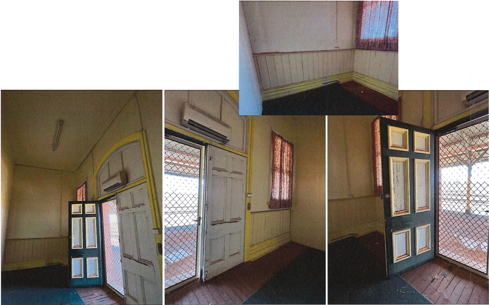
Photos 53, 54, 55, 56 Interior: entry off the platform into waiting room showing partition on the west side (left); doors detail and floor damage. Inset- dado detail.
