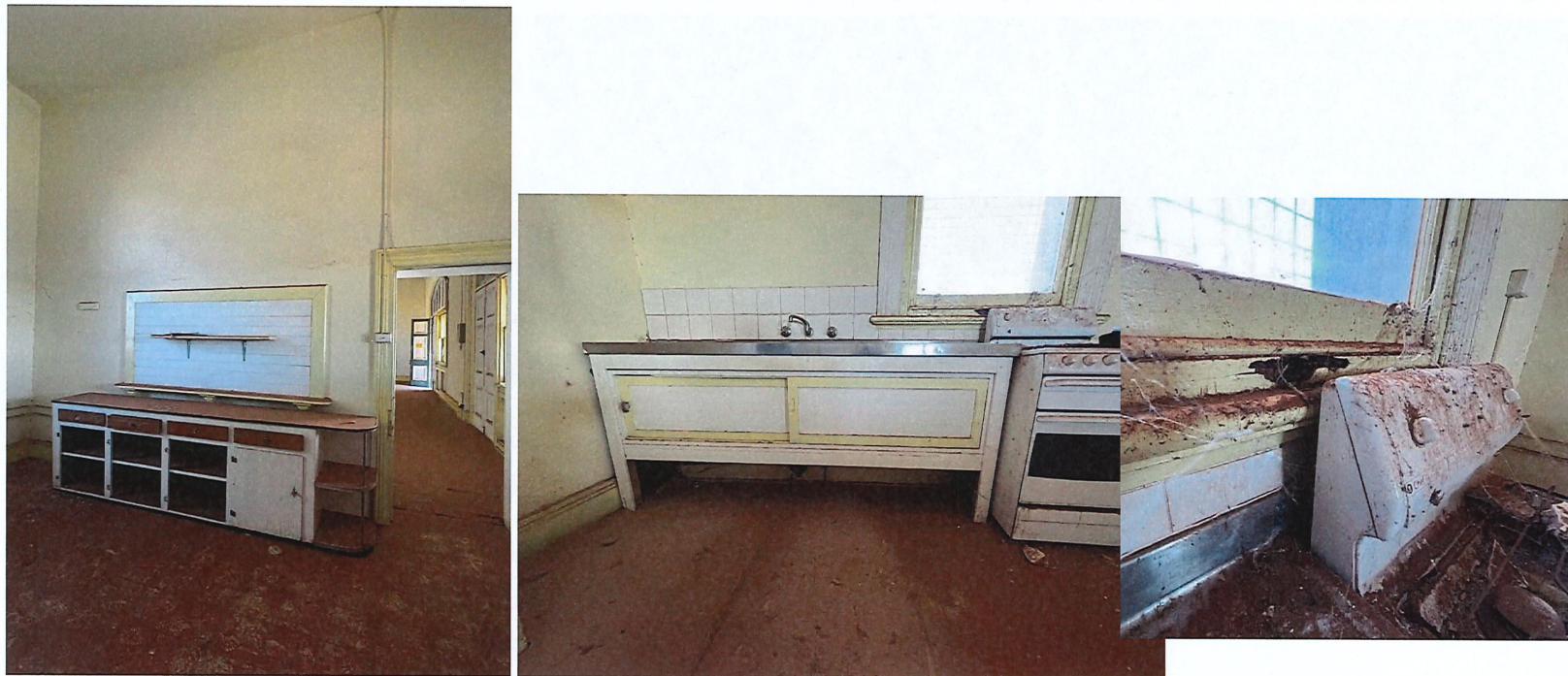
Photos 76, 77, 78, 79 Interior: kitchen showing north wall to Refreshment room, fireplace on south wall; sink unit and stove, and termite damaged window frame on the west.
