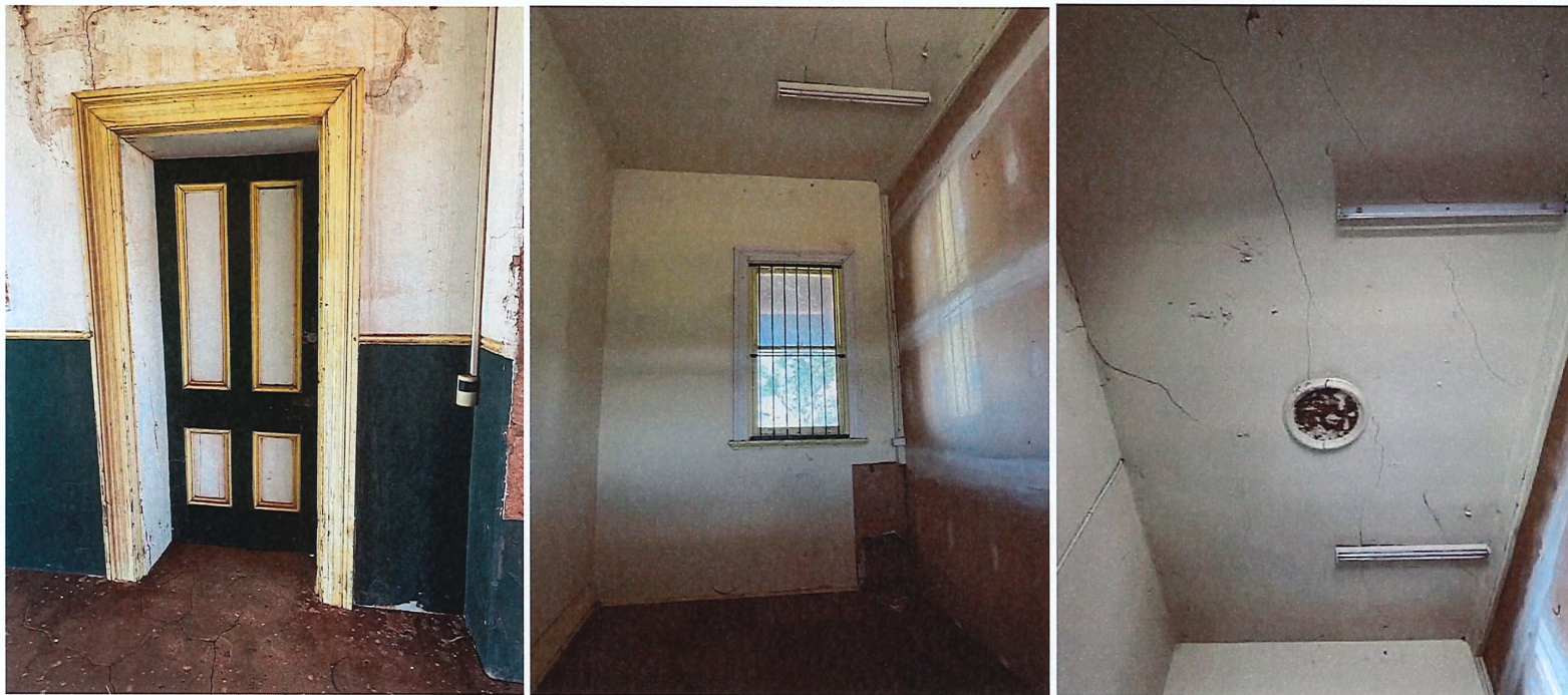
Photos 57, 58, 59 Interior: Door off luggage entrance into Ticket office showing west wall and gyprock north wall, and ceiling detail.
