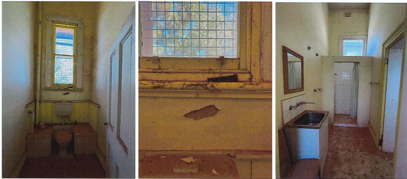
Photos 50, 51, 52 Interior: Ladies room toilet and detail of timber and wall damage (west wall), and laundry and shower (east end).
