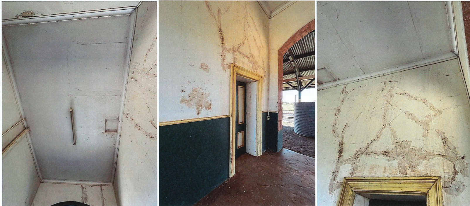
Photos 22, 23, 24 Views in the luggage entrance showing the ceiling, door to the ticket office and detail of the wall condition above that door.
