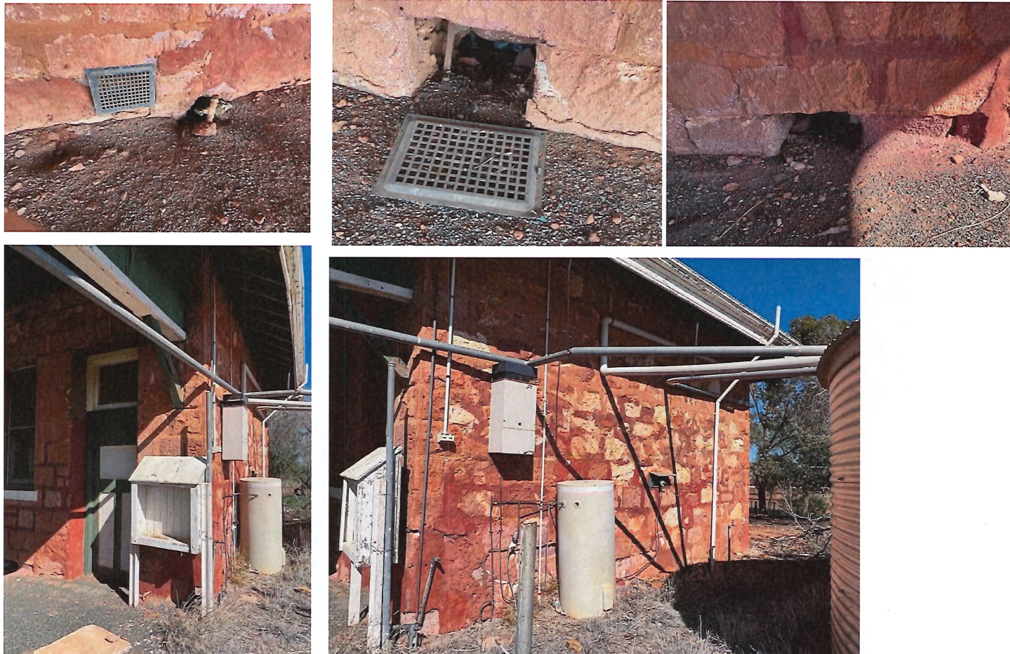
Photos 39, 40, 41 Examples of vents and vent openings along the base of the platform wall.
