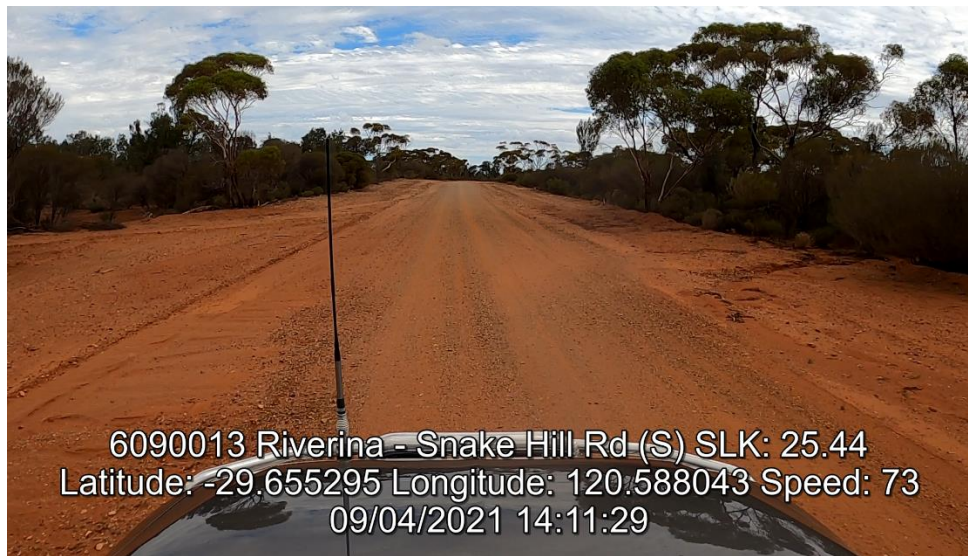
Post Damage Photo (After Photo 76)
