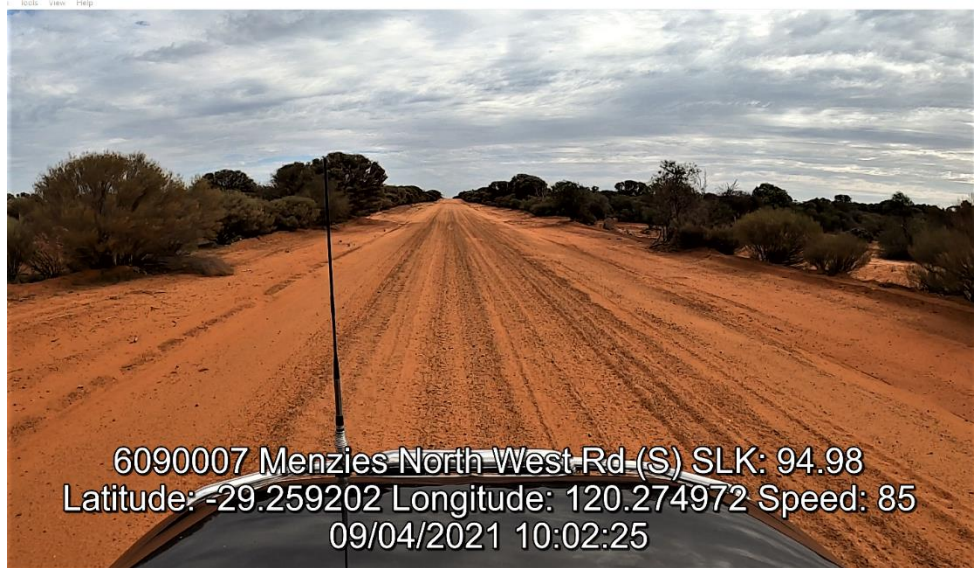
Post Damage Photo (After Photo 204)
