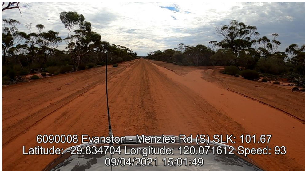
Post Damage Photo (After Photo 60)
