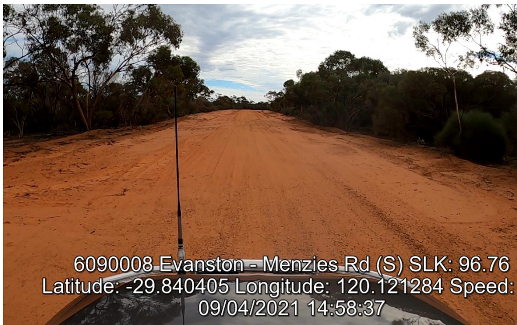
Post Damage Photo (After Photo 53)
