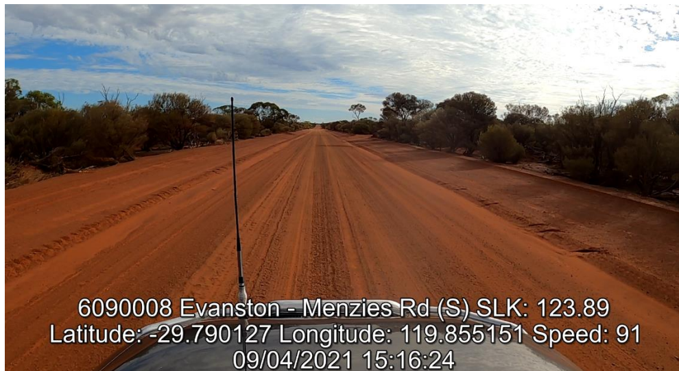
Post Damage Photo (After Photo 76)
